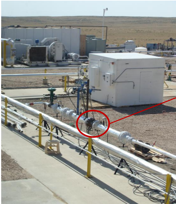
Gas Flow Testing – CEESI - Ft. Collins, CO USA
